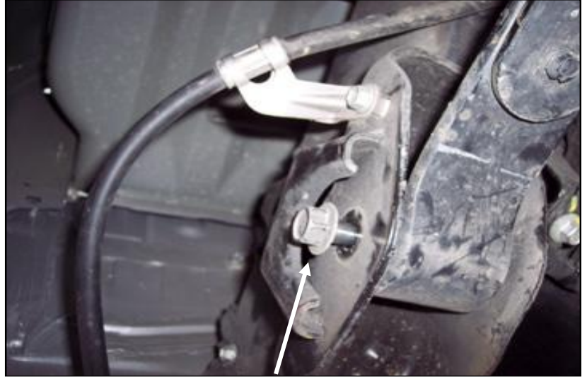
Factory bolt backed out 1/2"
