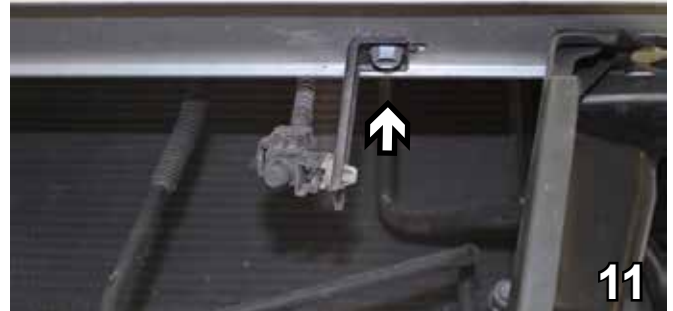
11. Beneath metal bumper, remove bolt for temperature sensor bracket with 10MM socket. Detach sensor from bracket. Set aside bracket and bolt to be reinstalled later.
