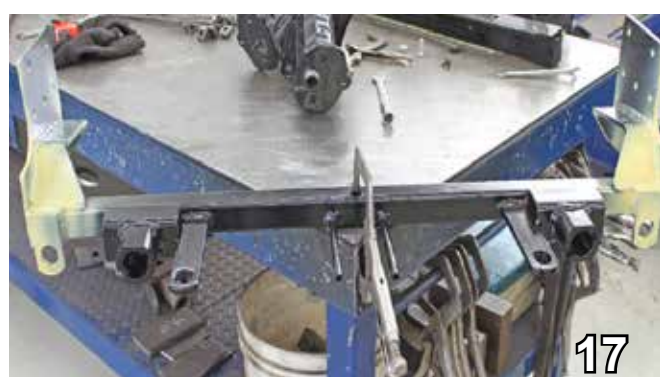
17. Lay baseplate in upright position on a smooth work surface (yellow is used on this baseplate for demonstrative purposes only). Anchor baseplate to work surface with vice grips.
