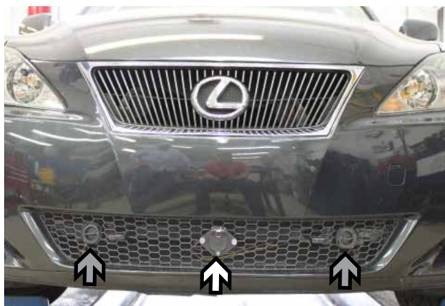
30. Reinstall foglights and connect sensor back onto fascia. Align the fascia to its original position and trim the opening for the attachment tabs with diagonal cutters (gray arrows). Do this on both sides of the vehicle. Optional: Attach the electrical bracket to the center of the fascia (white arrow). - Photo at left.
