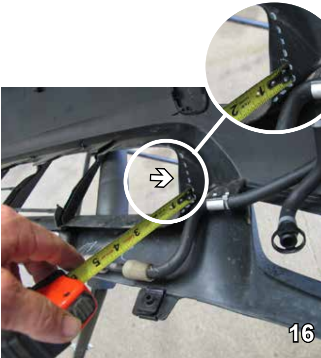
16. On the edge of the fascia opening, trim an inch in and taper back to the corner as shown. Do this on both sides.
