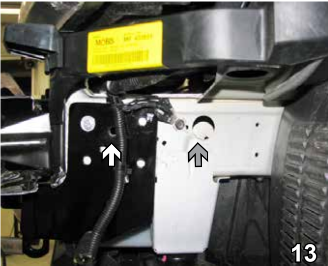
13. Using a 13/32" drill bit with the base plate as a template drill one hole (white arrow). Using a 1 1/4" hole saw, drill a hole in the frame next to the ground wires for the nut plates (gray arrow). Do this on both sides of the vehicle. Be sure to install only one bolt assembly per side to stabilize baseplate before drilling the remaining holes.
