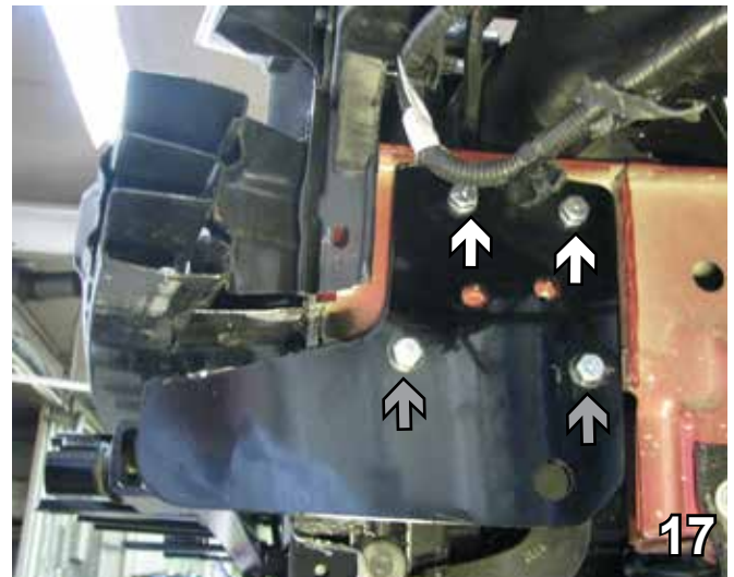
17. Using the baseplate as a template, drill the rest of the holes using the 13/32" drill bit. Insert 3/8-16 x 1 1/4" hex bolts with Loctite in all the holes. In the top two holes (white arrows), attach 3/8" lock washers and tighten to 3/8" nut plates inserted into the frame. In the bottom two holes (gray arrows), tighten to 3/8-16 nylon insert hex nuts. Do this to both sides of the vehicle.
