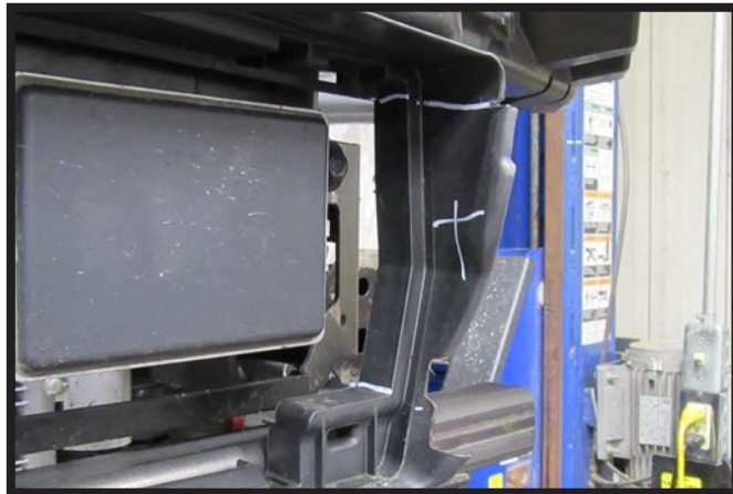
13. Using a reciprocating saw, trim the marked area on the driver's side shutter.
